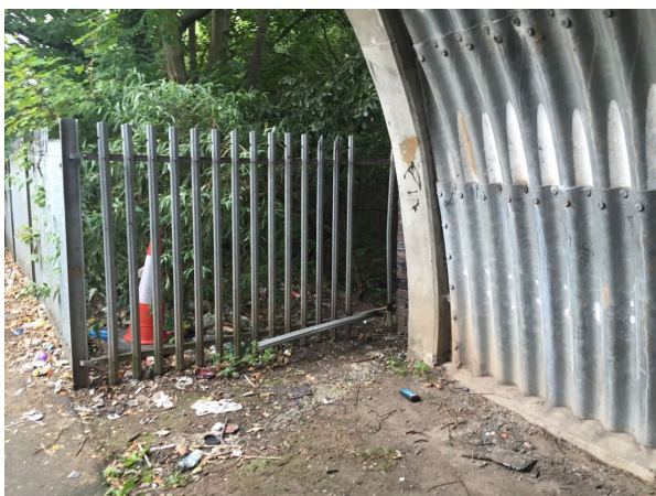
Figure 9 - 20 September 2016 12:55pm Damaged fence
